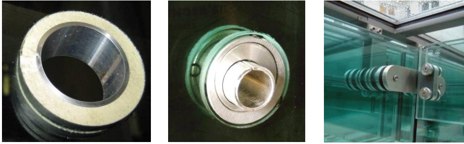
Figure 1a, b and c: Mortar-Interlayer to create ductility behaviour and example of a joint (CCI Munich)
